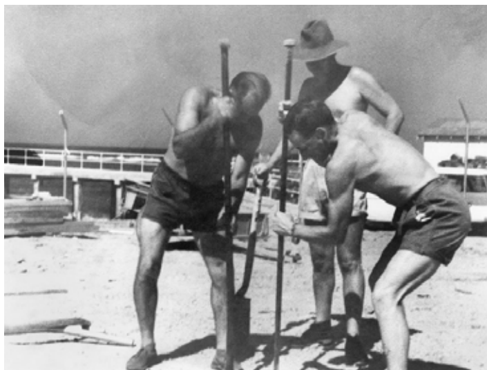
Above: Digging the first hole for the clubhouse in 1961, Sandy Alsop, Len Wilson and Rex Baldry.
