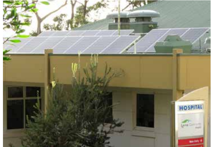
Above: A few of the many panels on the Lorne hospital. Image: Mary Lush
