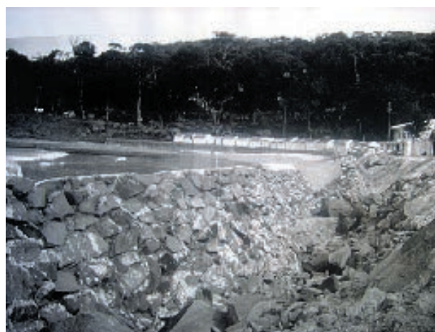
The destroyed seawall after the big blows of 1958.
